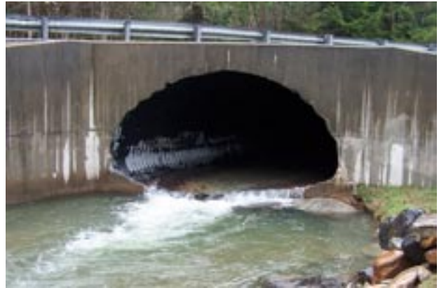
Perched culvert at Cummington Road (Riverways photo)
